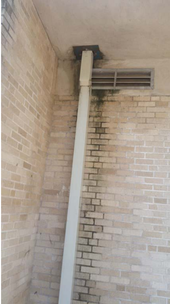
Roof leaks at gutters
