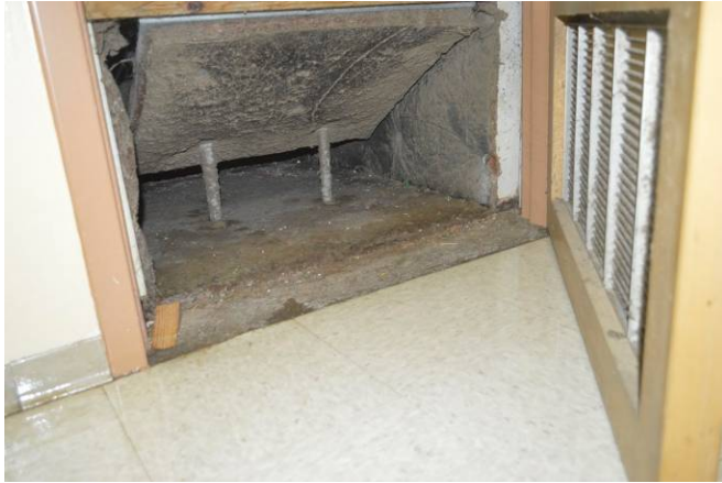
Flue rust and soot
