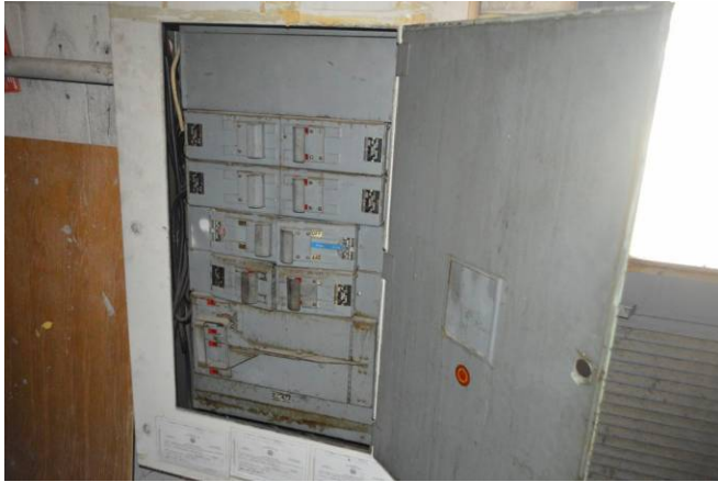
Older electrical panel box
