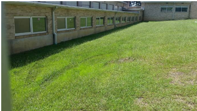
Slope of grounds is toward several buildings in areas
