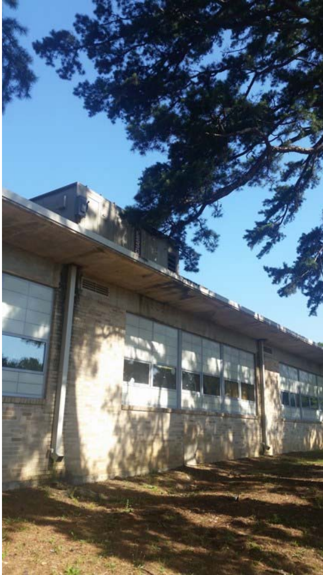
Roof leaks at soffit
