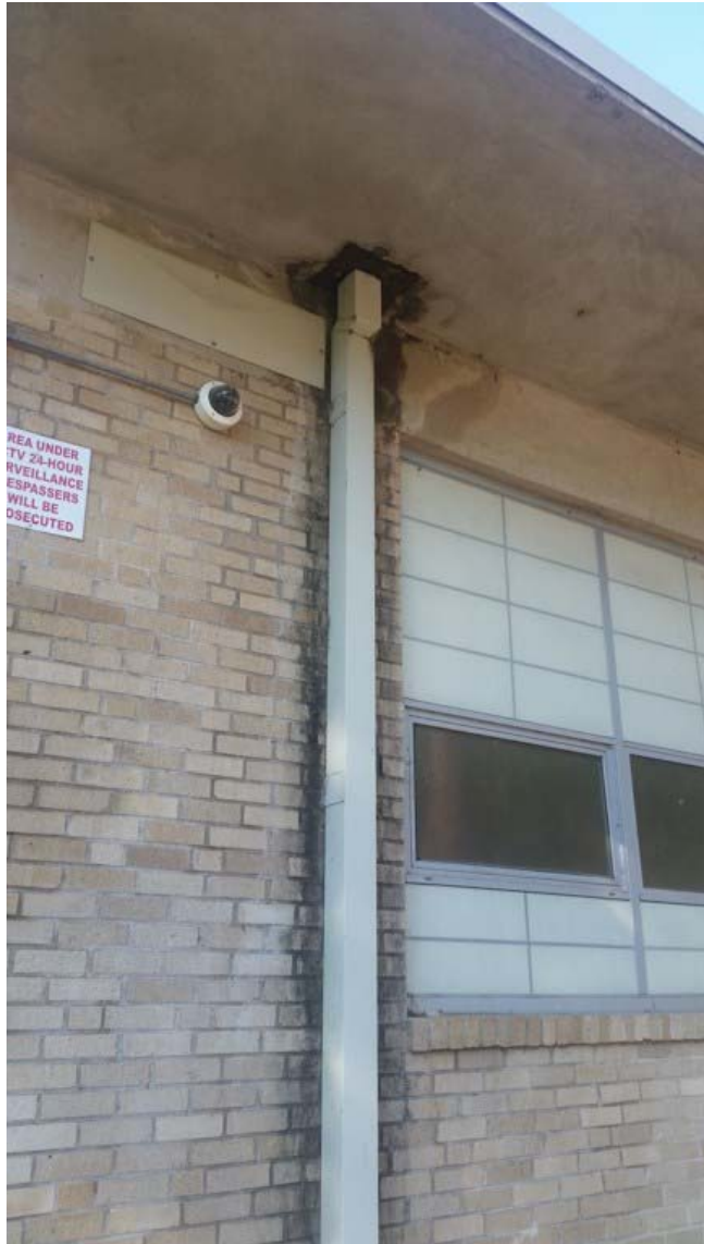
Roof leaks at gutters
