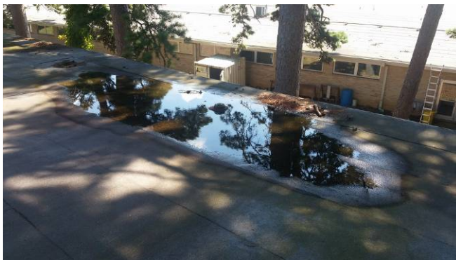
Example of ponding on roof
