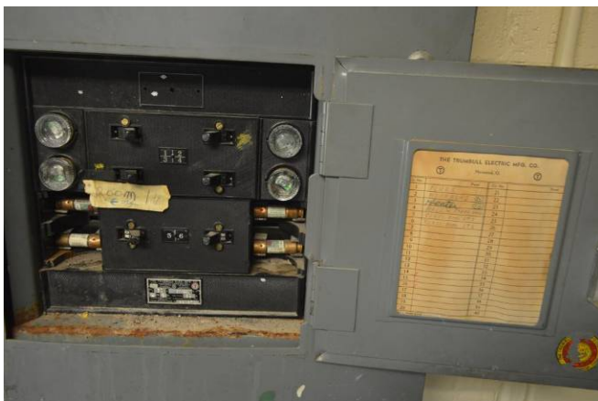
Older electrical panel box
