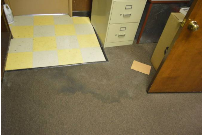
More water stains
