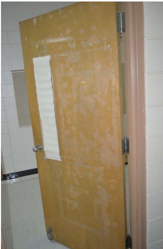
Door surface damage example
