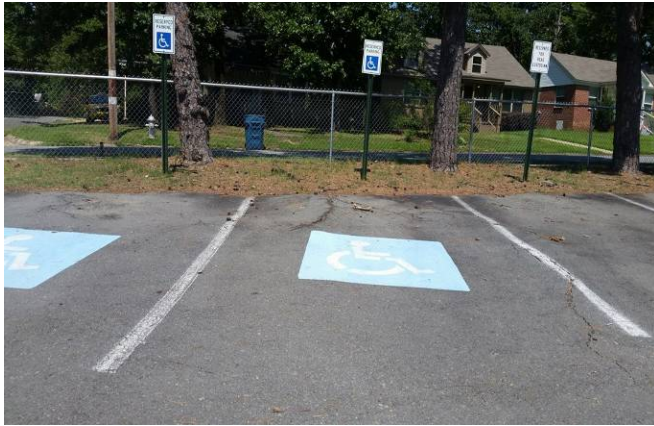
Parking lot wear
